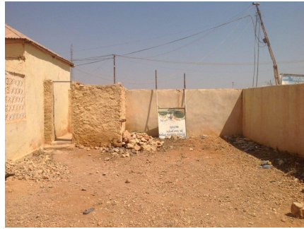
View of existing latrine. It has no roof or entrance door.
