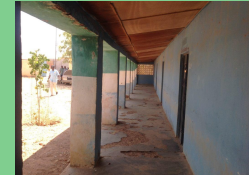
The floors are in worn condition, columns and beams are chipping.
