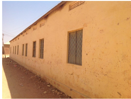
The existing structure has walls along the parcel boundary with windows opening to the outside of the compound.
