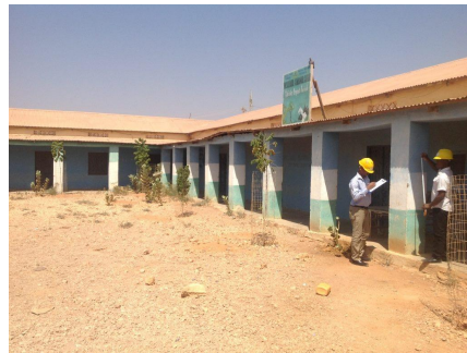
The roof is in worn condition.
