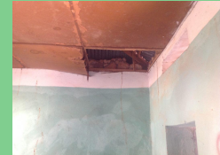
The ceilings are in worn condition.
