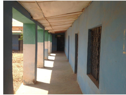
23no. columns, of 400X400mm, run along the corridor that serves the rooms.
