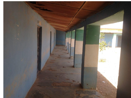
Columns are bent, beams are sagging.
